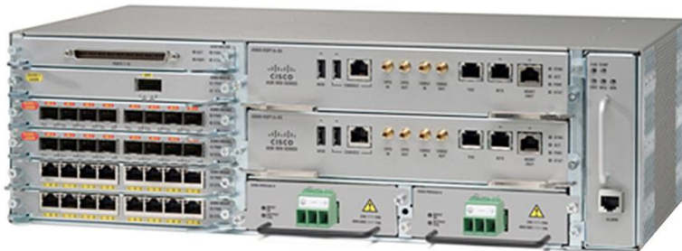
Figure 3: Cisco ASR 903 Router
